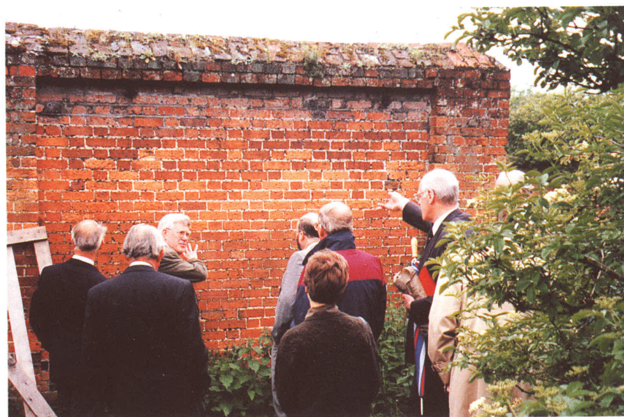
Members of the Livery with guests being shown the damage caused by masonry bees in an 18th century wall at Painshill Park. It was part of a one day Seminar on Joints and Jointing of Brickwork - one of a series of seminars organised by the Craft Trust to promote a better understanding of the crafts of tiling and bricklaying.
